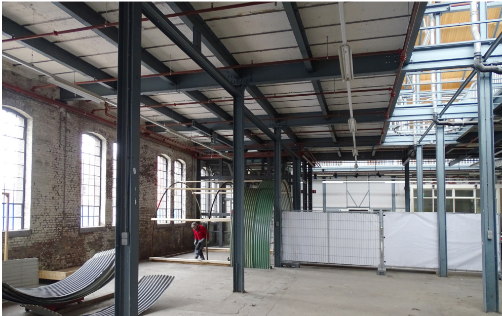
View from the big hall on the ground floor, showing the primary, secondary and floor construction.
