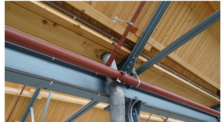
Close up of rainwater drainage system.
