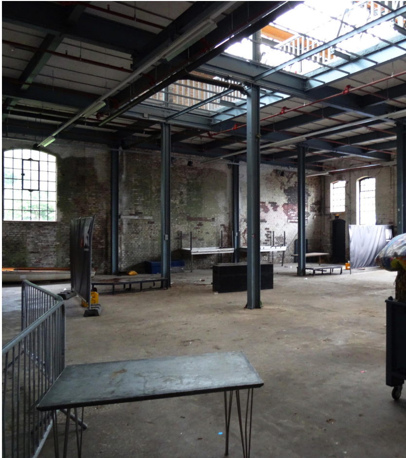
Looking to the north at the big hall on the ground floor, showing the high space, visible structure, voids and daylight..
