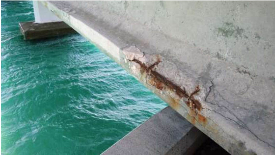
Figure B. 3 RC member affected by reinforcement corrosion [9]
