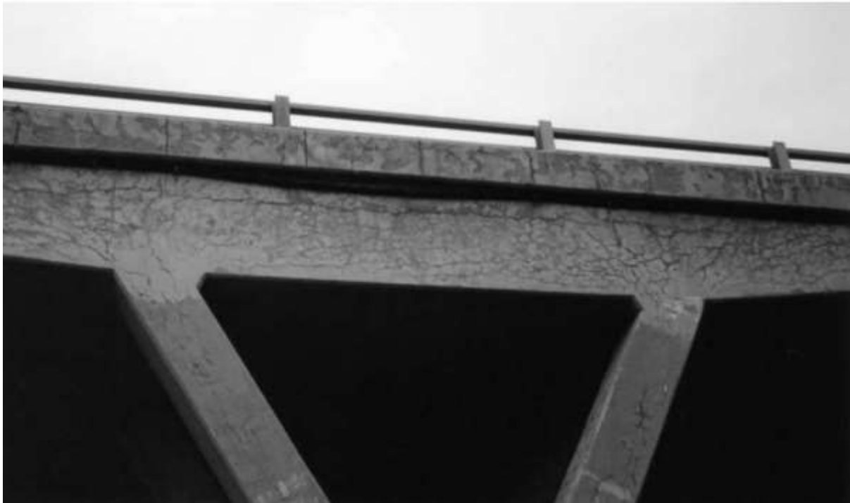
Figure 1. 2 Map-cracking due to alkali-silica reaction and cracks preferentially oriented along the main reinforcement [7]
