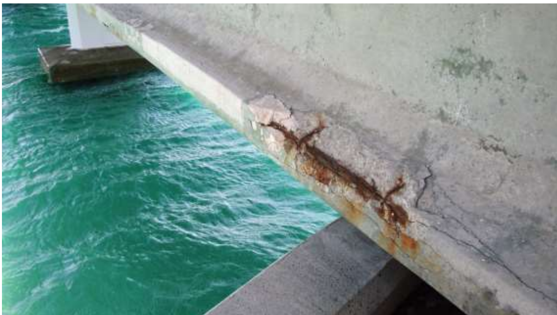
Figure 1. 4 RC member affected by reinforcement corrosion [9]
