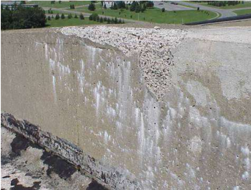
Figure B. 5 Surface scaling of concrete due to freeze-thaw cycles [11]
