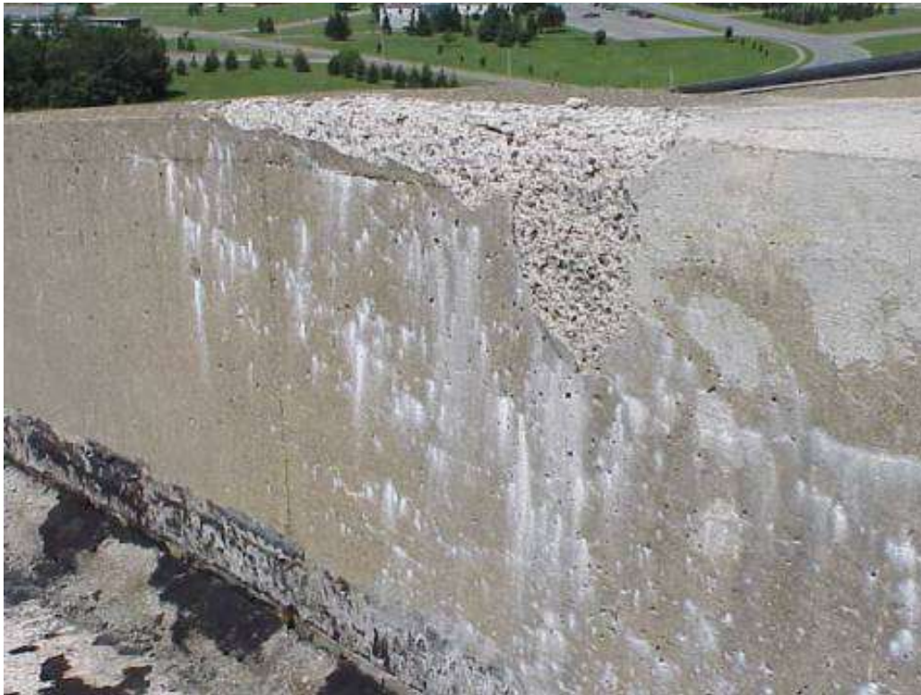
Figure 1. 6 Surface scaling of concrete due to freeze-thaw cycles [11]
