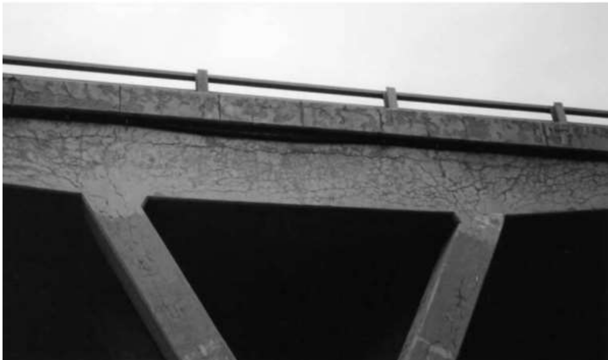
Figure B. 6 ASR map-cracking and cracks preferentially oriented along the main reinforcement [7]
