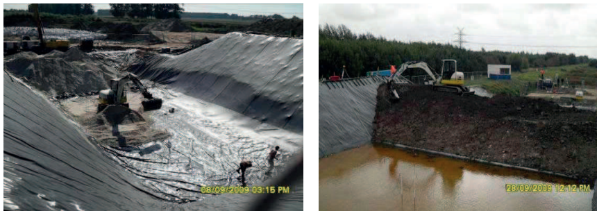
Figure 8 and 9 Filling the basins with sand (left) and building the clay levee (right)
