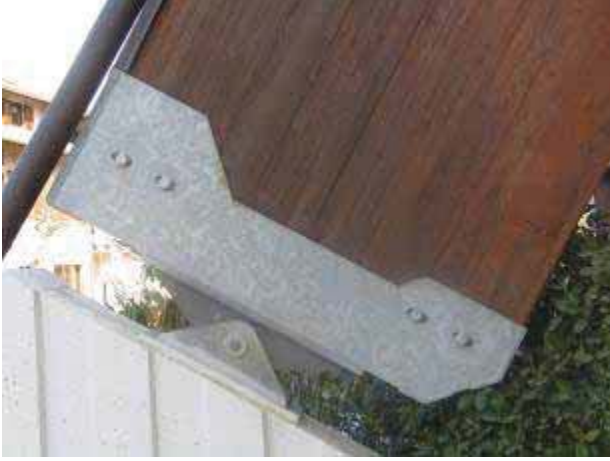
Figure 3: Cracked glulam beam in outdoor climate. Cracks occur where the maximum shear stresses are expected.
