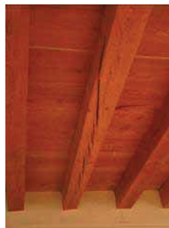
Figure 2: Cracked beam in a historical structure
