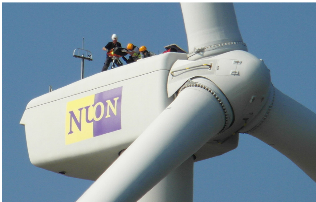
Figure 37: Onno, Chris and Erik installing the Wind Iris on top of the turbine
