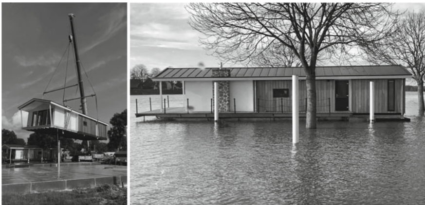
Fig. 5 Chalets with aluminium foundation during construction and afloat during floods (source Resort Marina Oolderhuuske)
