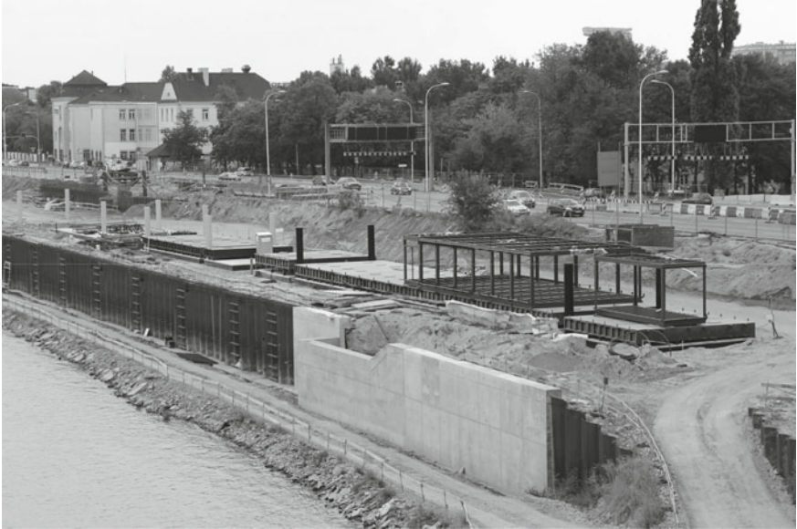
Fig. 8 Construction process on the amphibious pavilions in Warsaw in June 2017. Dolphin piles, concrete foundations, and steel pontoons are visible (image taken by author)
