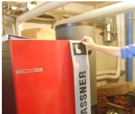
FIGURE 8.10 IEWAN: Collective pellet heater
