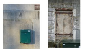
6. Filling of the basement entrances and windows with brickwork and finished with a concrete plaster
