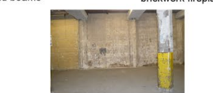
9. Removal of the old elevator and addition of new yellow brickwork walls
