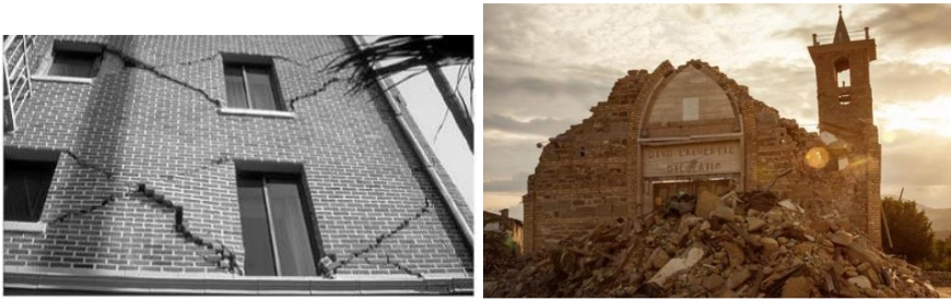
Figure 1.2: Damage in masonry structures due to earthquakes, taken from [2, 3].
