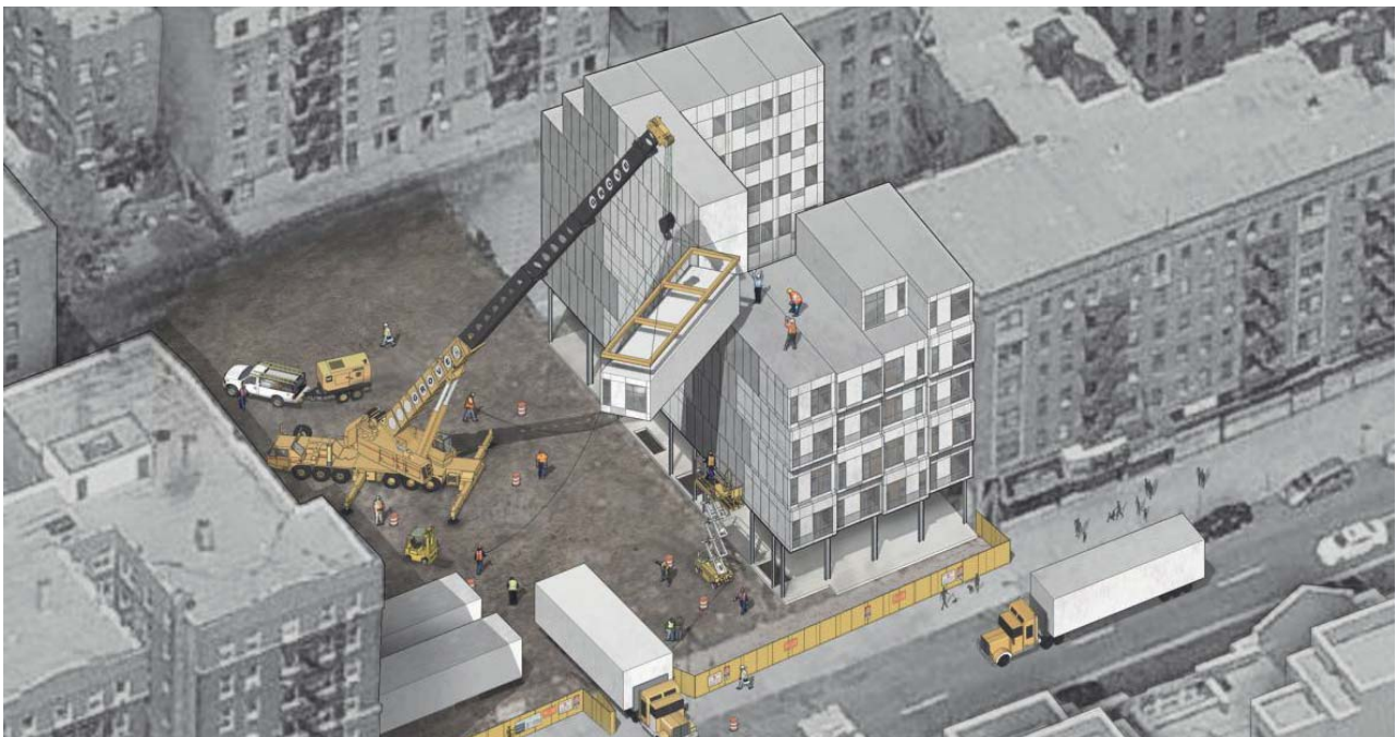
Figure 1 - Installation of the module took 19 days, an eight person crew and a crane
