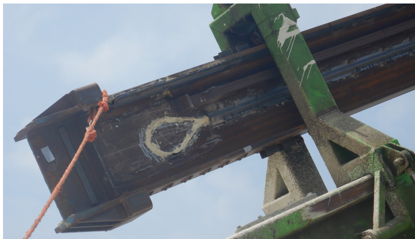
Figure 2.9: Photo of MV test pile illustrating the loop configuration of BOTDA sensor and protection by a welded steel bar (personally taken photograph: Putteman, J.).
