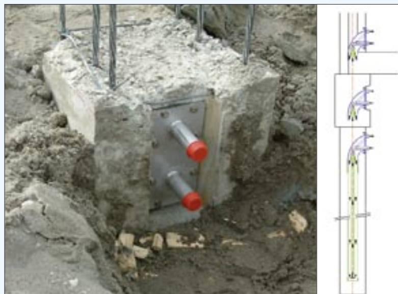
Another option is to use special piles doubling as heat exchangers. The heat extracted from the earth is fed through a closed circuit inside the pile to the heat pump.
