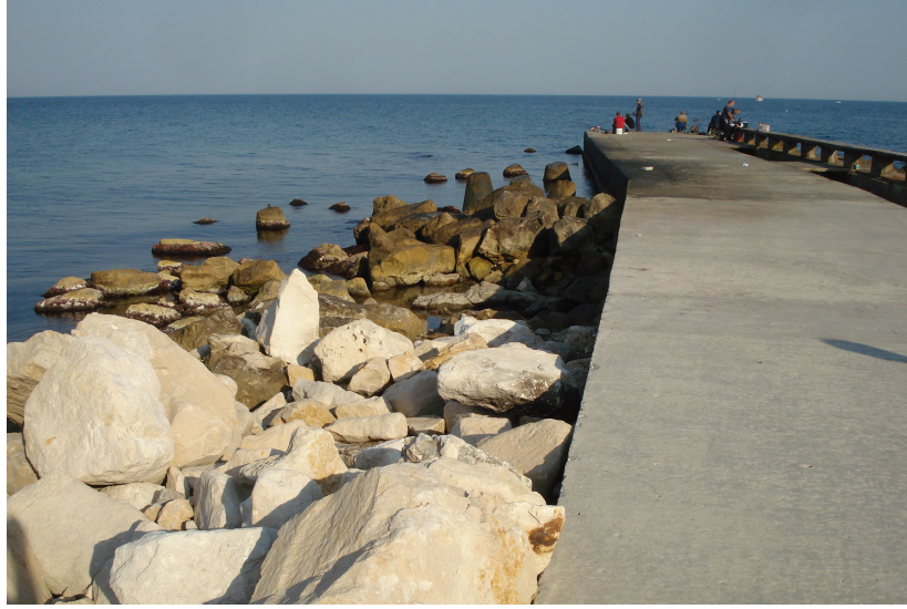
Figure 1.2: Example of damaged breakwater, Asparuhovo breakwater, Bulgaria
