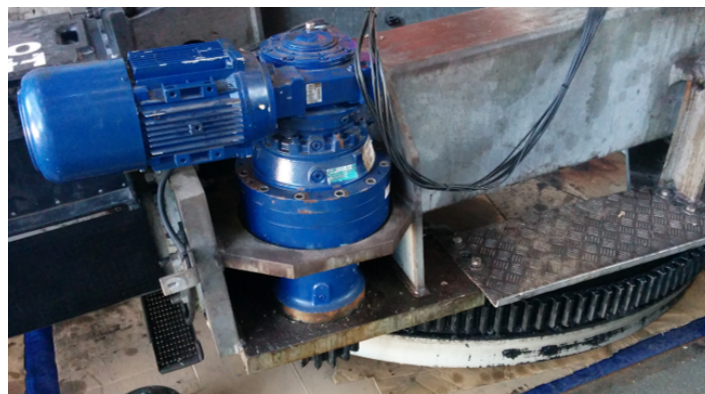
Figure 2-27: One of the two yaw motors driving the small pinion gear against the large bull gear of the bearing, which connects the nacelle frame to the tower.
