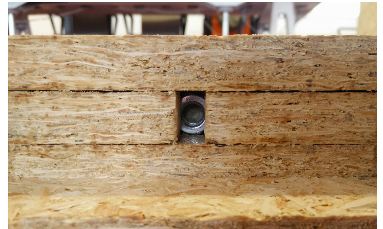
Figure 8.8 Inaccuracies of the inserted nut at the bottom and top of the floor (Own illustration)
