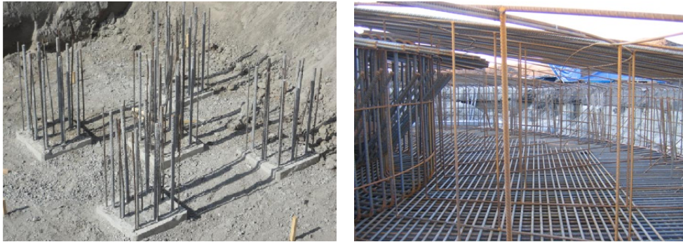
(a) Uncovered pile reinforcement [49]
