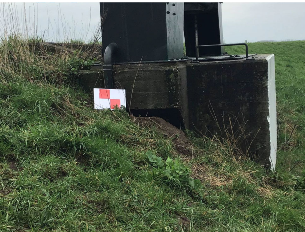
Figure 9. Example of the presence of multiple damage parameters at a single damage point (4_3). At least bare spots, weeds and rough vegetation could be applicable here, while the cause of the bare spot (just right of the reference marker) could be burrowing.
