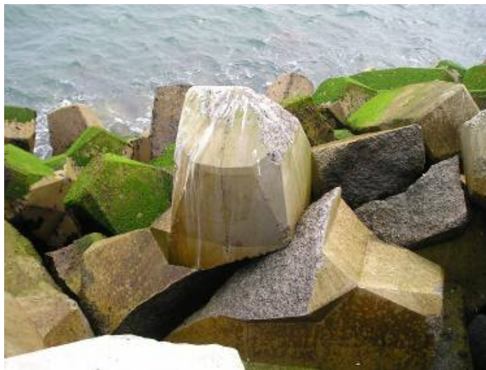
figure 2.2: Broken Accropode unit at the damaged seawall of Scarborough, UK
