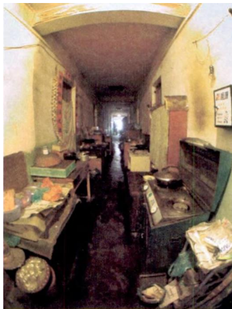
Figure 4. A dim Corridor in a Tongzilou with cooking utensils and other stuff left by various residents. (Xia and Yin, 2007)
