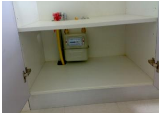
Figure 12. Gas meter in kitchen, hidden in the cabin. (Qijia, 2018)
