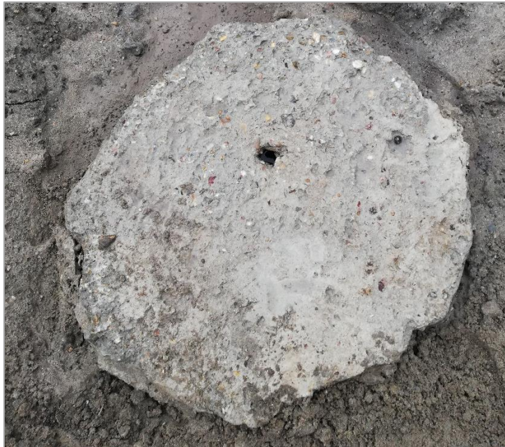
Figure 5.2: Conduit in hardened concrete resulting from excessive bleeding ( D_{\text{conduit}} \approx 30\text{mm} )
