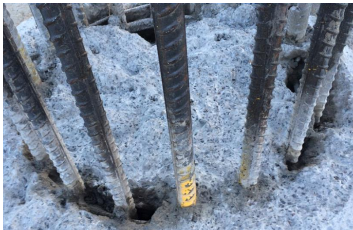
Figure 5.3: Bleed water travelling upwards along reinforcement bars (From Larisch, 2019)
