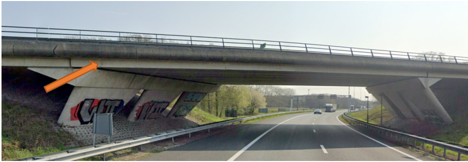
Figure B2.1: 'Grollegat' viaduct in connecting road between A65 and A58 motorways near Tilburg, the Netherlands. The orange arrow points at the location where the core are drilled. Source: Google Streetview
