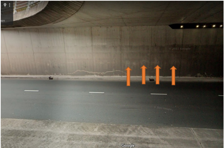
Figure B2.10: Location of core drillings (marked with the orange arrows). Source: Google Street view
