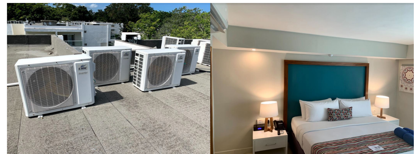
Figure 48: Condensators and evaporator units (split) as cooling energy technology used in the Hotel Emotions. Source: own
