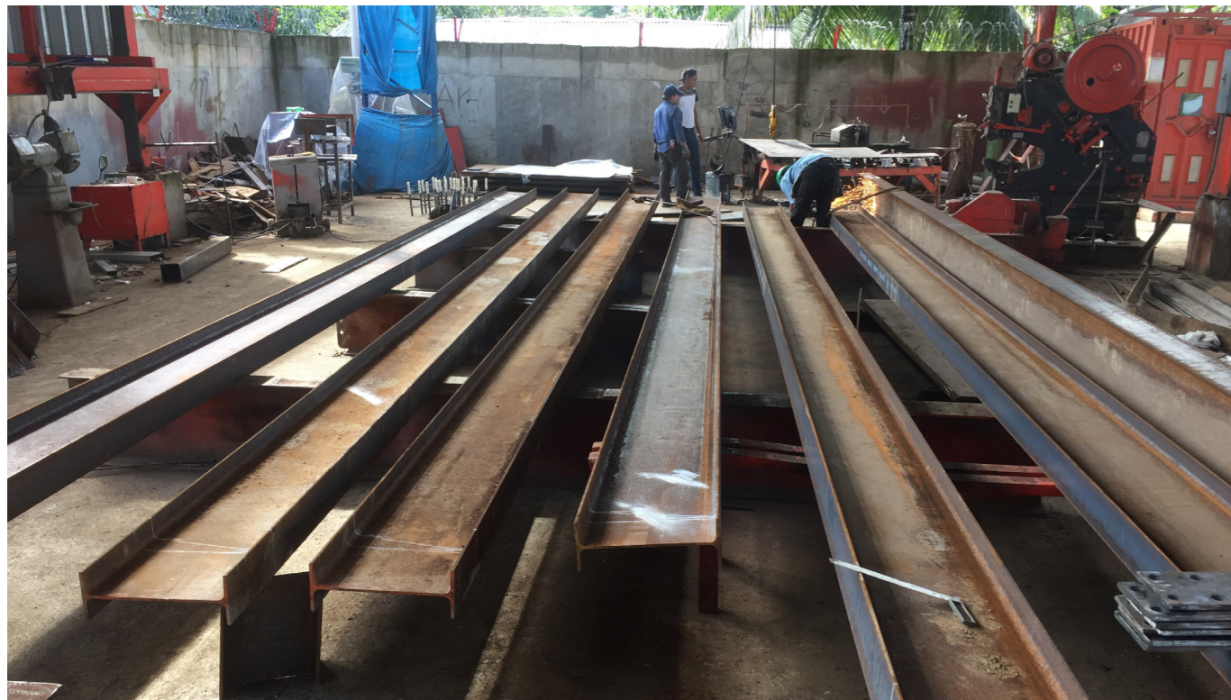
Figure 46: Practical examples of steel beams inside a workshop. Source: own
