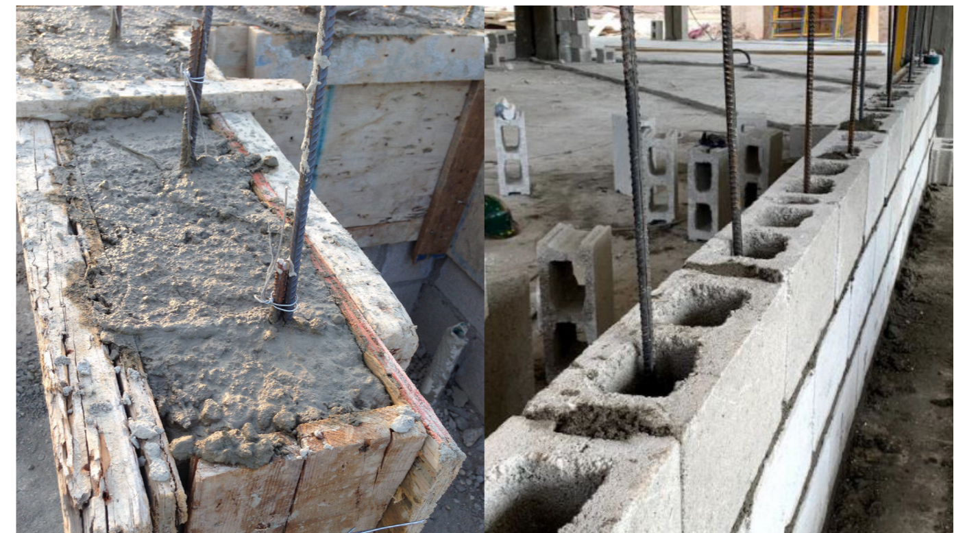
Figure 44: Practical examples of cast-in concrete and block mampostery in the construction of a coastal hotel in Jamaica. Source: own
