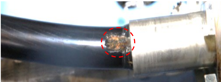
Figure 63: Part of the defective joint showing clearly the degradation of the insulation screen.
