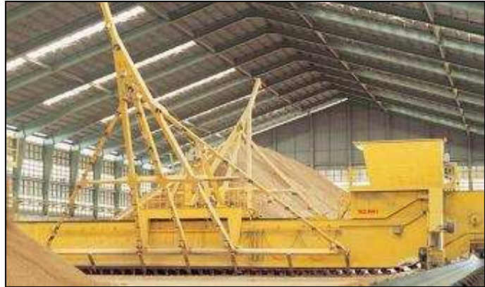
Figuur 2.5b: bridge type scraper reclaimer
