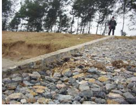
Figure 4.9: Failure of revetment at transition
