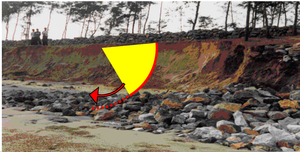
Figure 4.5: Heavy damage of revetment and outer.
