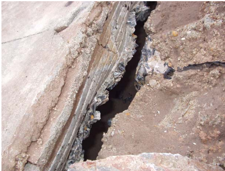
Figure 4.9 Failure of filter layer at Vanly section
