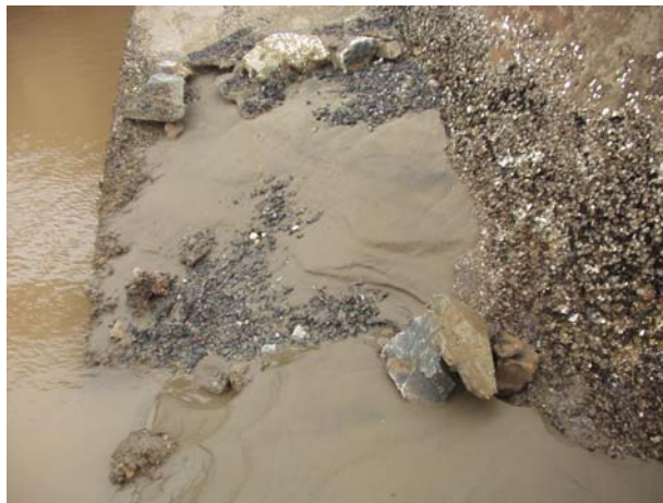
Figure 4.8: Damage of cover layer, the filter layer exposures ( Haichinh section )
