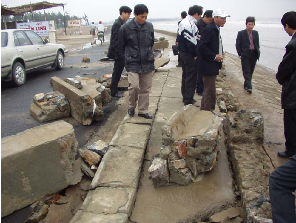
Figure 4.3: Damages of crest-wall at Namdinh seadike at Haithinh section
