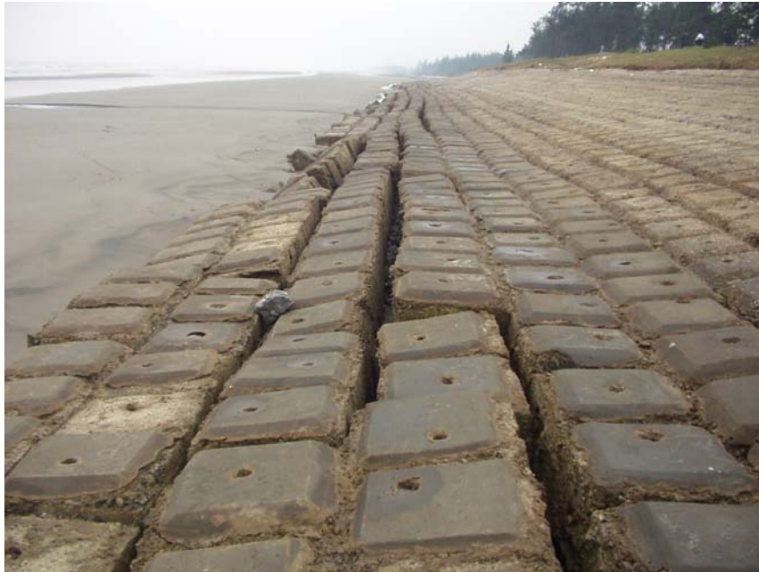
Figure 4.10: Failure of toe structure leads to damage of revetment (HaiTrieu section)
