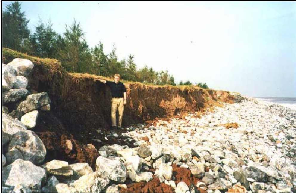
Figure 2.7: Severely eroded dike with planted casuarinas trees at HaiHau beach.
