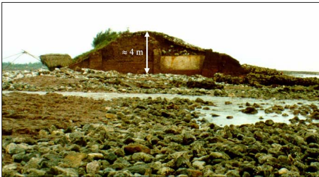
Figure.2.8: Characteristic cross-section of an eroded dike near VanLy village
