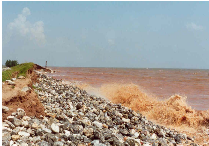
Figure 1.1: A damaged dike section
