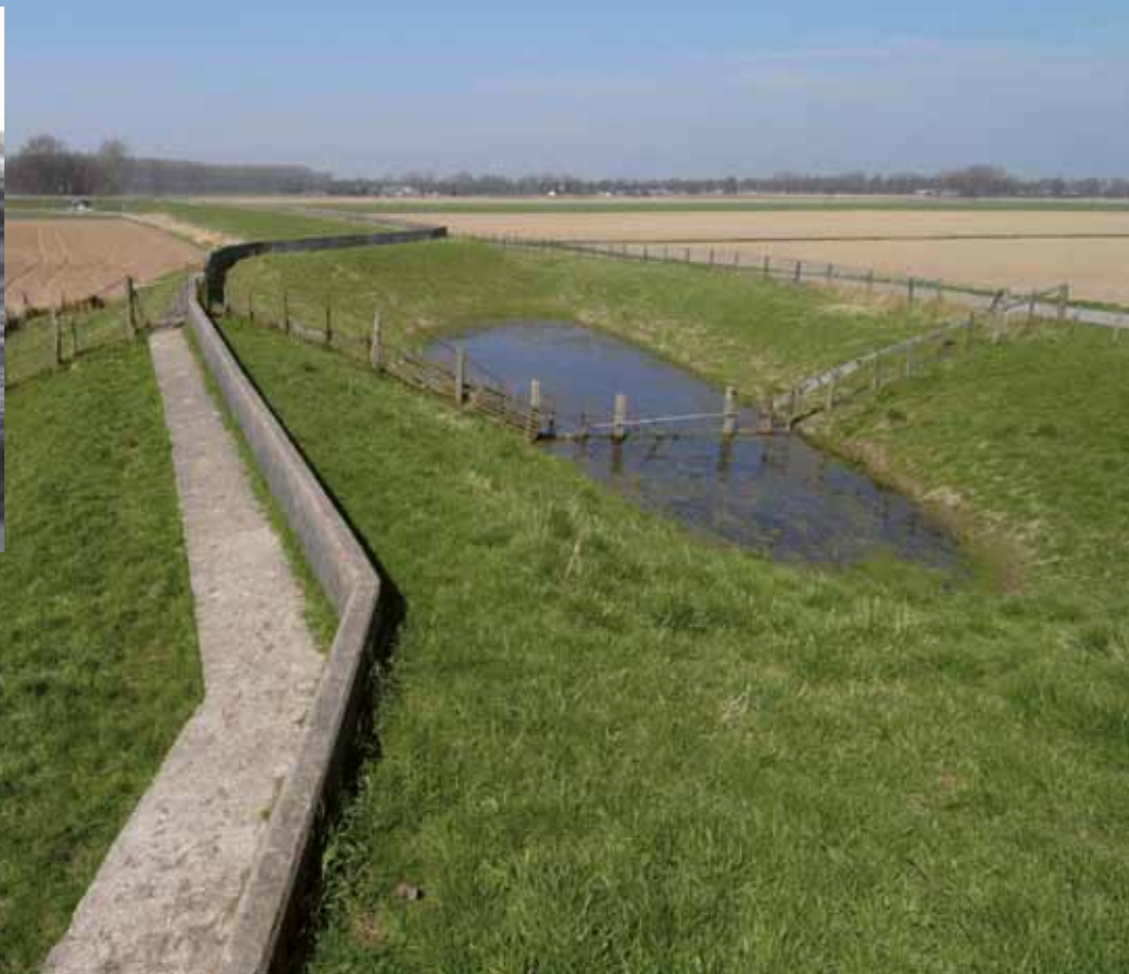
Muralt wall on the Schenkeldijk at Werkendam. Countless dykes in Zeeland were reinforced with these walls between 1906 and 1939. Most have since been removed.
