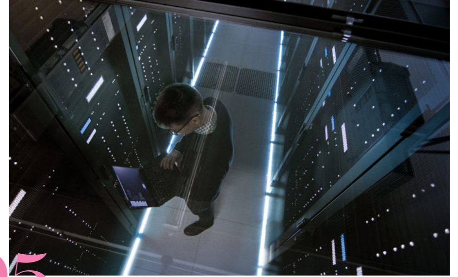
Fig. 3.18, Data Center Data centers serve as the main physical hardware infrastructure for the cloud layer. Image source: https://www.mdac.tw/news_20210706_1
