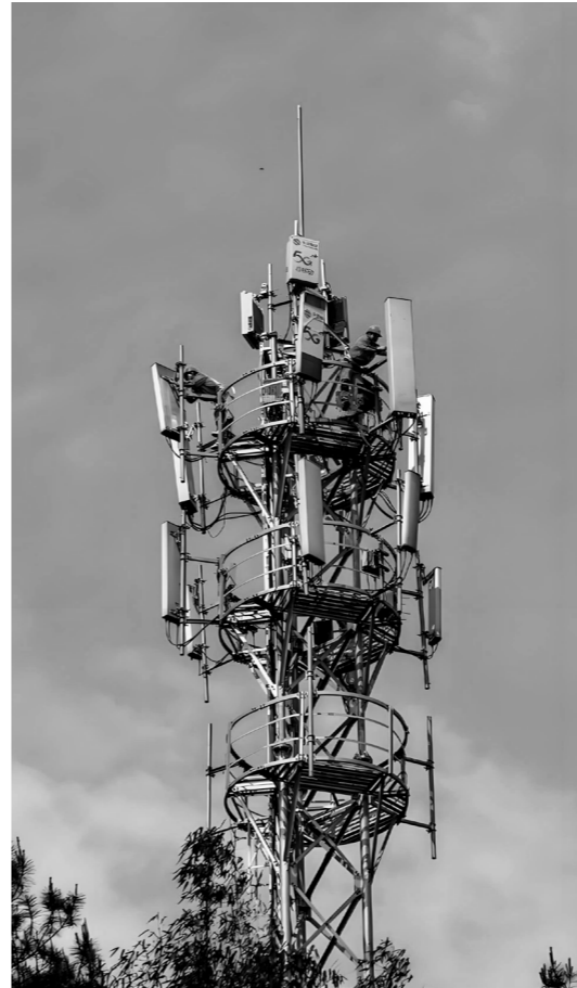
Fig. 3.16, Cell Tower Cell towers provide wireless connectivity between users' devices and the broader cloud network. Image source: https://bbs.zhyoo.com/zhyoo/208931.html
