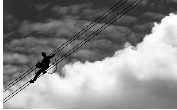
Fig. 3.5, Electrical lineworker at height Extensive manpower in power grid construction in western China. Image source: https://opinion.caixin.com/2020-06-16/101567851.html
