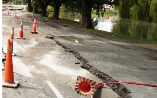
Figure 2. Lateral spreading beside lowland rivers.
