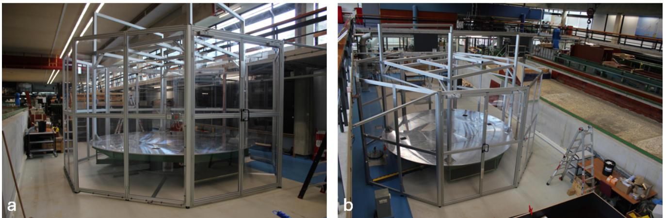
Figure 3: Photographs of the completed construction, including the turntable, overhead frame and the safety fence: a) viewed from the lab floor, b) viewed from the upper floor balcony.
