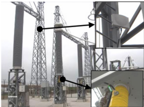
Fig. 3. Overview of one side of a 380 kV cable system. The top inset shows the antenna which is used to make the wireless communication with the main computer and other measuring units possible. The lower inset shows a detail of the internal inductive PD sensor.
