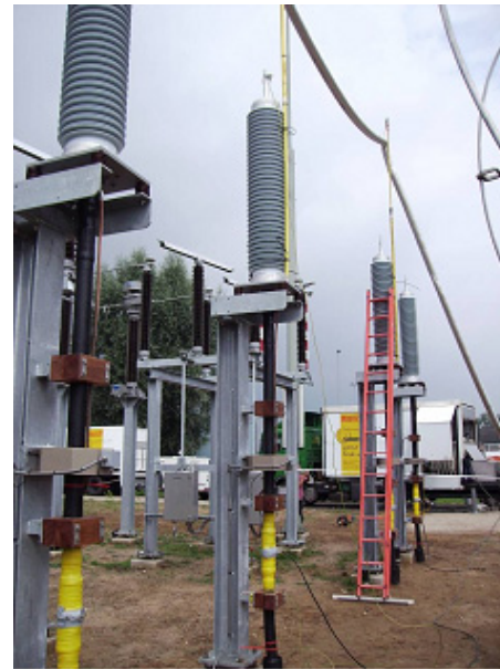
Fig. 7. On-site testing of two 2-phase 150 kV cable systems with integrated inductive PD sensors.
