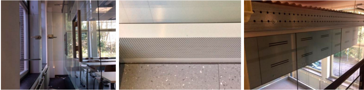
FIGURE 3.5: Natural ventilation (left), displacement ventilation: plinth for air supply at the long sides of the room (middle) and exhaust through the ceiling (right) (Bluyssen et al., 2017). Used with permission from the author.
