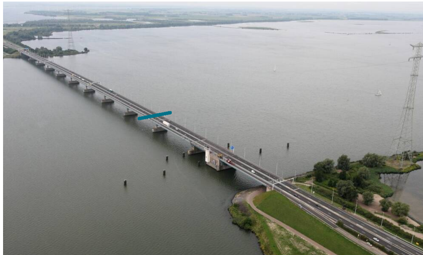
Figure 3.4: Aerial picture of the Haringvlietbrug. The approximate location of the sensors is indicated in cyan (source original picture: Rijkswaterstaat).
