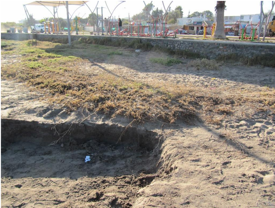
Scour at the beach side of the road
