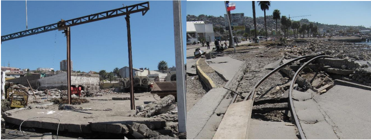
Only entrance structure remained, trucks pushed together and railroad tracks were bend.
