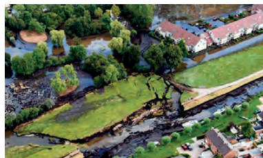
Figure 2: Regional levee breach in Wilnis in 2003 caused by drought. (Source: AFP, 2003)
