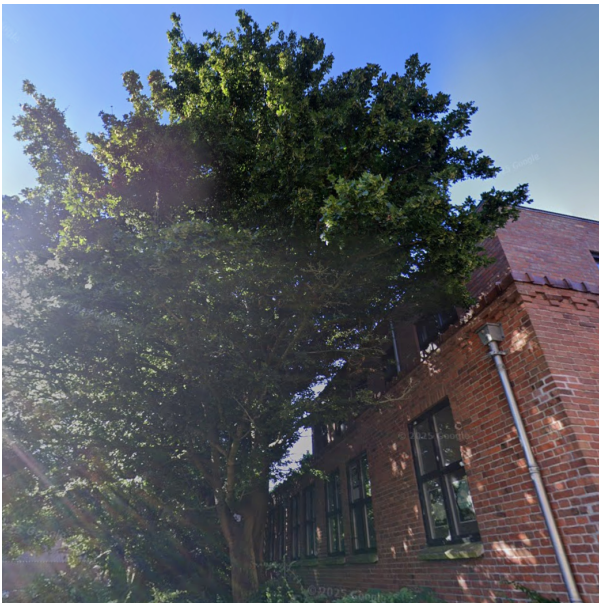
(a) Street-level view of the test site showing the tree canopy in direct contact with the building façade.
