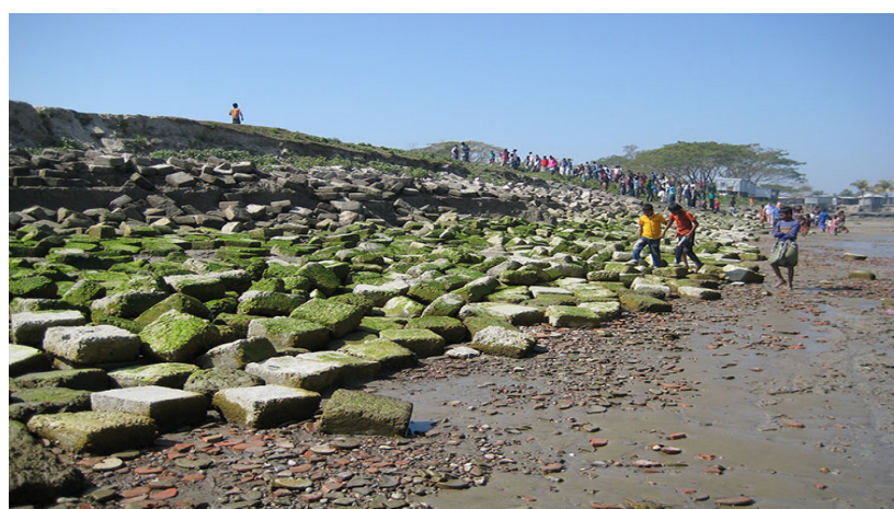
Figure 2.10. An eroded Dyke on the Island of Bhola, Bangladesh. Retrieved from https://www.royalhaskoningdhv.com/nl-nl/nederland/nieuws/nieuwsberichten/20140625pb-nl-experts-ontwikkelen-kustbeschermingsplan-bangladesh/3333
