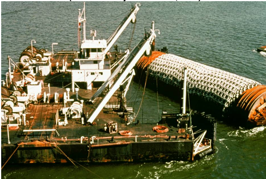
Figure 6.3 Bed protection equipment as used for the Eastern Scheldt barrier (Beeldbank Rijkswaterstaat, 1983)
