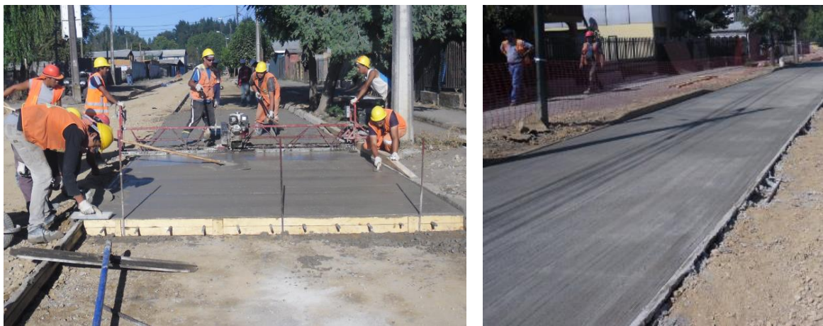
Fig. 5.5.1. Paving with fixed formwork (left) and general view of the test section (right).
