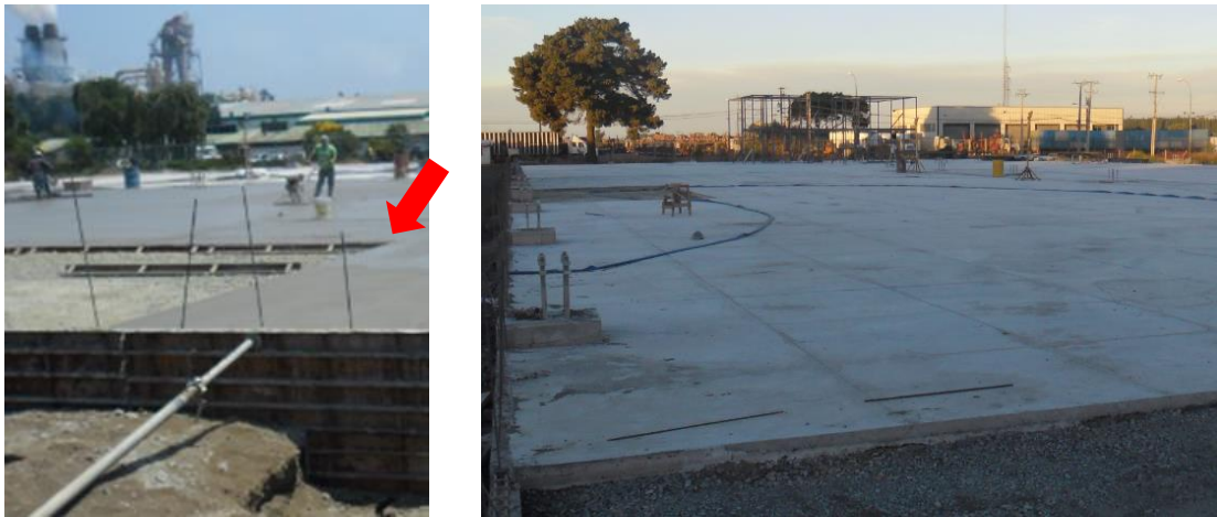
Fig. 5.5.3. Construction of industrial floor with shorter irregular sections (left) and general view of the industrial floor (right)
