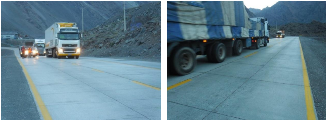
Fig. 2.2.1. Short slabs at the Route 60-Ch ‘Christ the Redeemer’, Chile.
