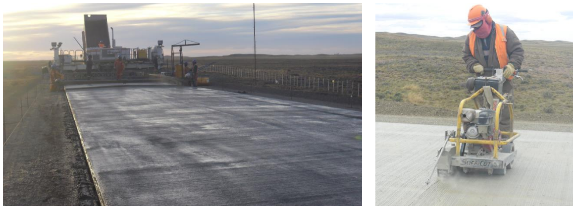
Fig. 5.5.2. Paving with slipformer (left) and (early-entry) saw-cutting of the transverse joints (right)
