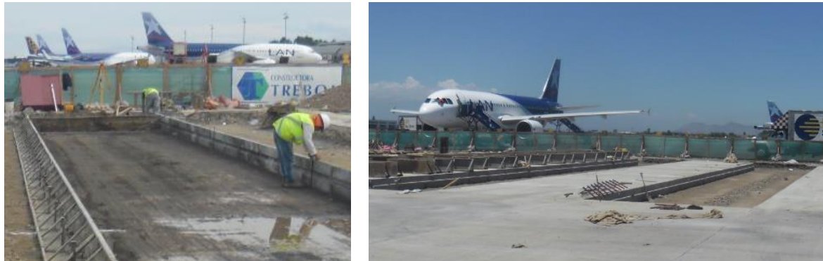
Fig. 5.5.4. Paving with fixed formwork (left) and general view of the test section (right).
