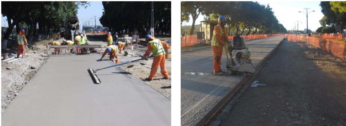
Fig. 5.4.4 Paving with formwork (left) and saw-cutting the transverse joints (right) of the Chilean JPCP.
