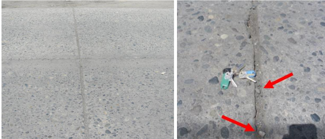
Fig. 7.3.4. JPCP with coarse incompressible material and spalling (joint width 20 mm).
