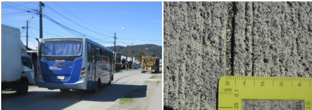
Fig. 7.3.5. Traffic and UnJs state in JPCP in a street in an ultra-high rainfall zone (saw-cut 3 mm) (Pradena & Houben, 2015a).
