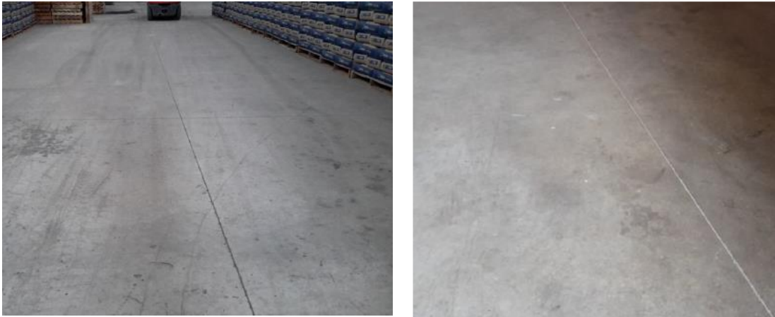
Fig. 7.3.11. General view of the industrial floor and an example of joint state (Pradena & Diaz, 2016)
