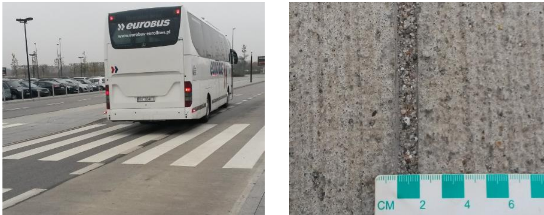
Fig. 7.3.3. Sealed joints contaminated with incompressible material at bus stop, Wrocław city, Poland.
