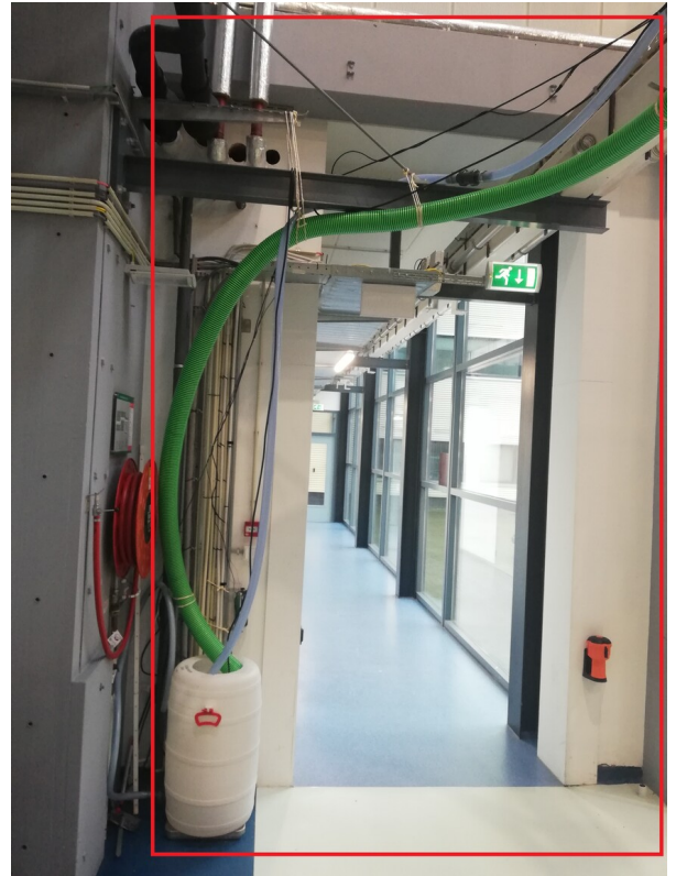
Figure A.6: End of the flowloop
