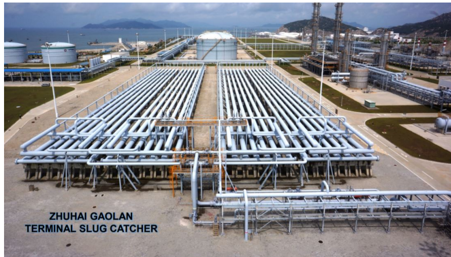
Figure 1.1: Zhuhai Gaolan Terminal slug catcher designed for a maximum of 44000 barrels ( \approx 5246 \text{ m}^3 ). Reproduced from Thronson [33].
