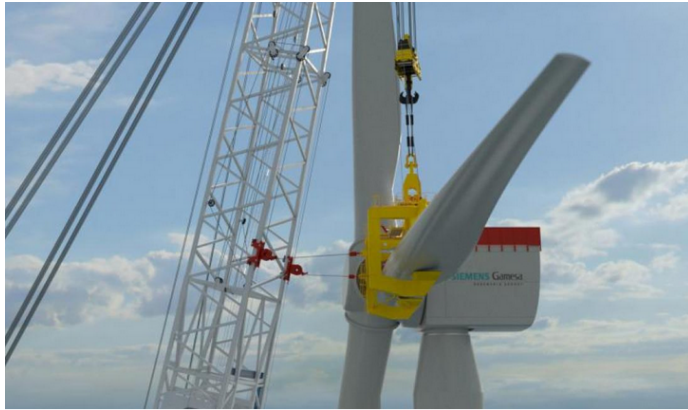
Figure 1.2: Tugger ropes connected to the load of a crane. These ropes can be used to reduce sway in crane operations.
