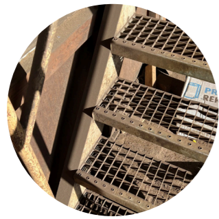
mesh on stairs
