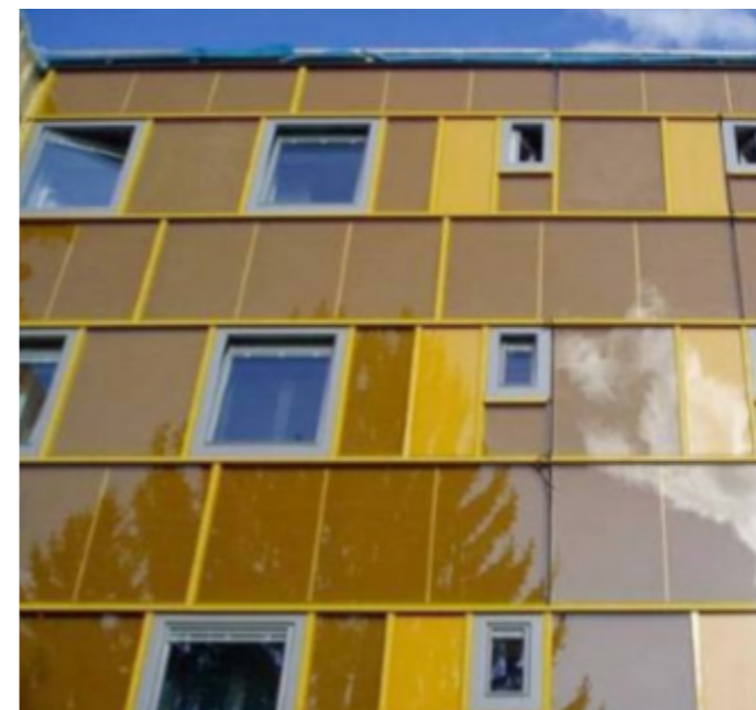
Figure 4 Cross section of new thermal envelope (top). Figure 5 Prefabricated facade module (middle). Figure 6 A view of the facade (bottom), (IEA , 2011).
