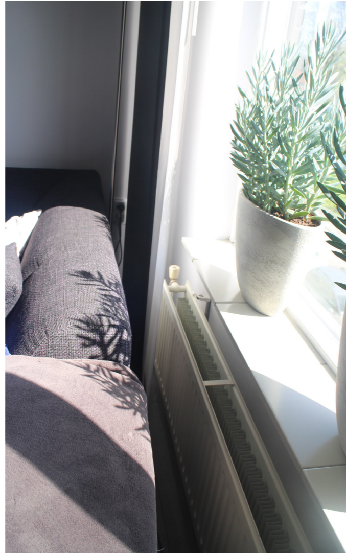
Figure 8 The radiator installed currently.(Source: KAW, 2017)
