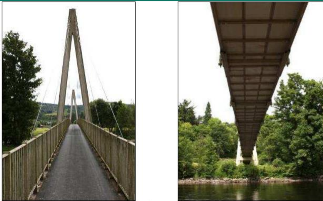
Figure 87: (Left) Deck and Tower of the Aberfeldy Footbridge, (Right) Bottom of Bridge Deck 117
