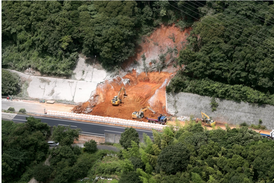
Figure 1-1 A landslide blocks the Kyushu Expressway [3]
