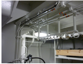
Figure 4.16: Pipe bundle which could have been produced on a frame in the workshop
