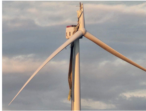
Figure 1.1: Damaged blade at the Vineyard Wind offshore wind project [32].
