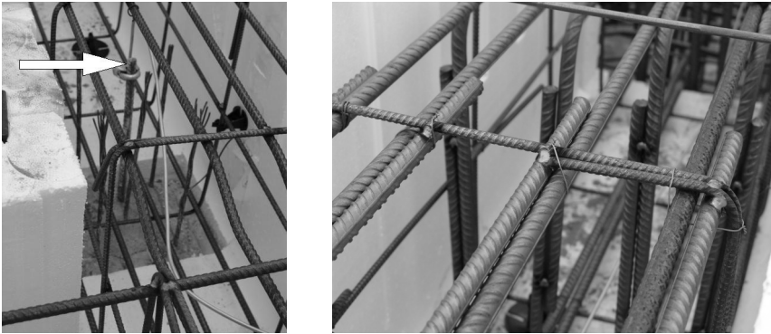
Figure 7.1: Left: Corner of foundation reinforcement. It can be seen that the reinforcement of the foundation is one big cage. The thick vertical rod in the middle of the pile (see arrow) is for grounding purposes. Right: Two ways of connecting reinforcement, welding or using iron wire.
