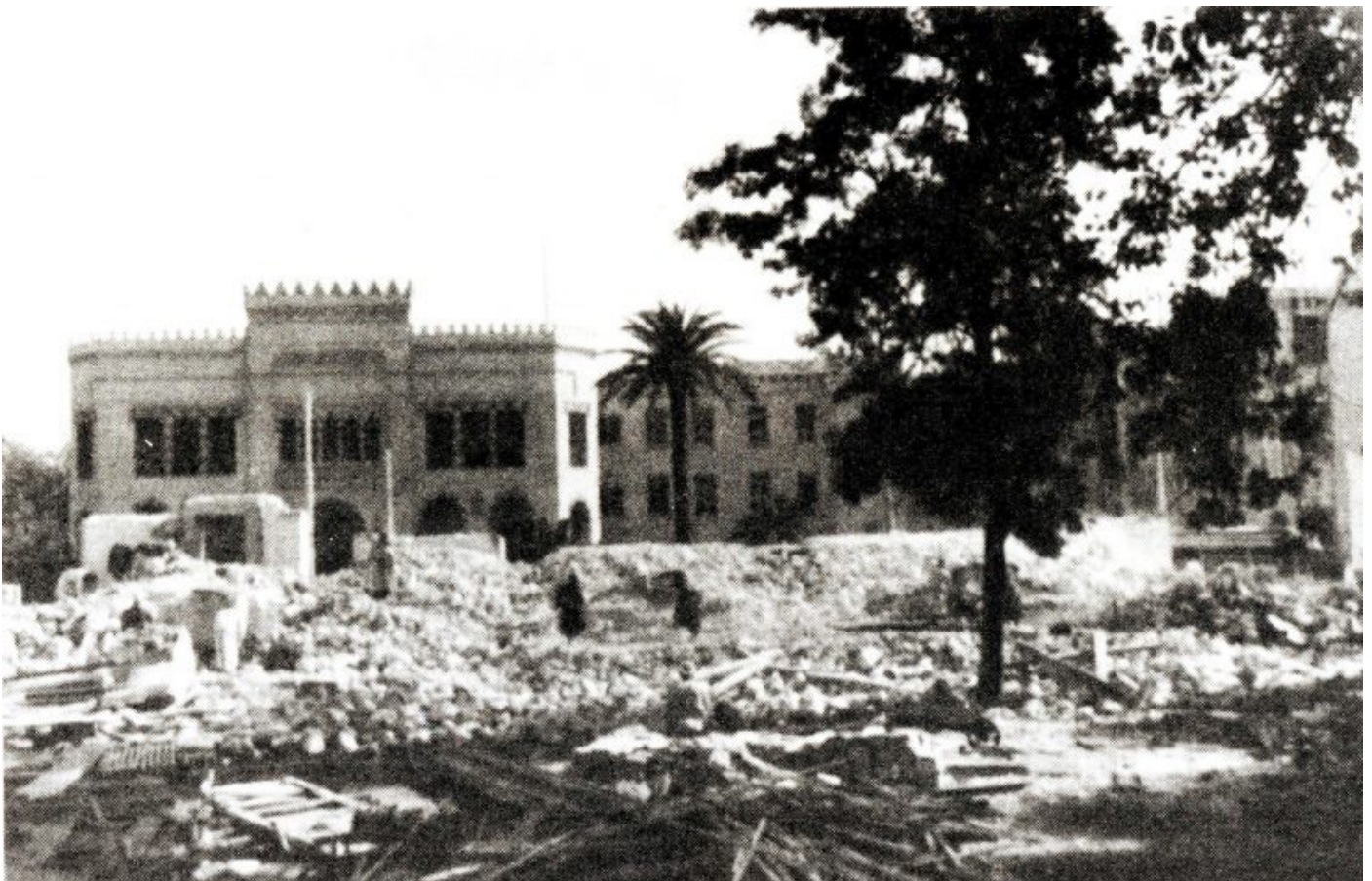
Figure 2.8: Ismailia Palace demolished with the AUC visible in the background. in 1938 (el Kolaly, 2011)
