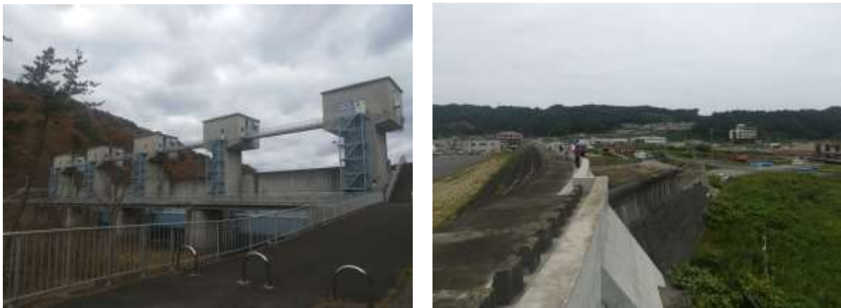
Figure 11. Left: dyke and floodgates at Fudai, which successfully stopped the force of the tsunami, despite being partially overtopped (inundation marks of ~20m in front of the structure). Right: coastal defences at Taro were overtopping by the tsunami, which went on to completely destroy the town behind them.
