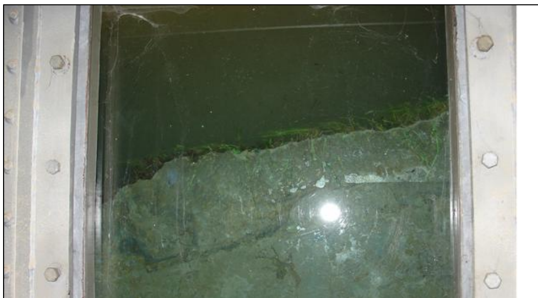
Figure A-18: Horizontal crack formation under a large section of the grass cover.
