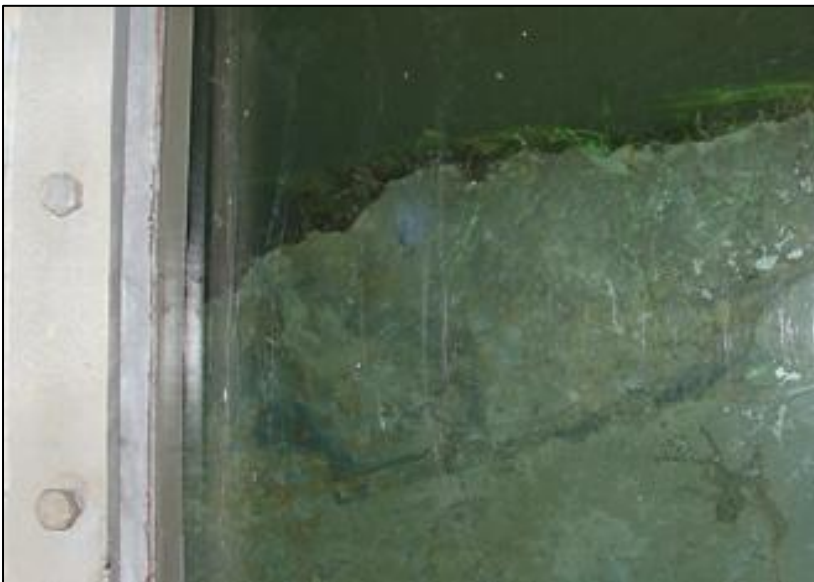
Figure 4-9: Horizontal crack formation in the wave impact zone during the EroGRASS experiments.
